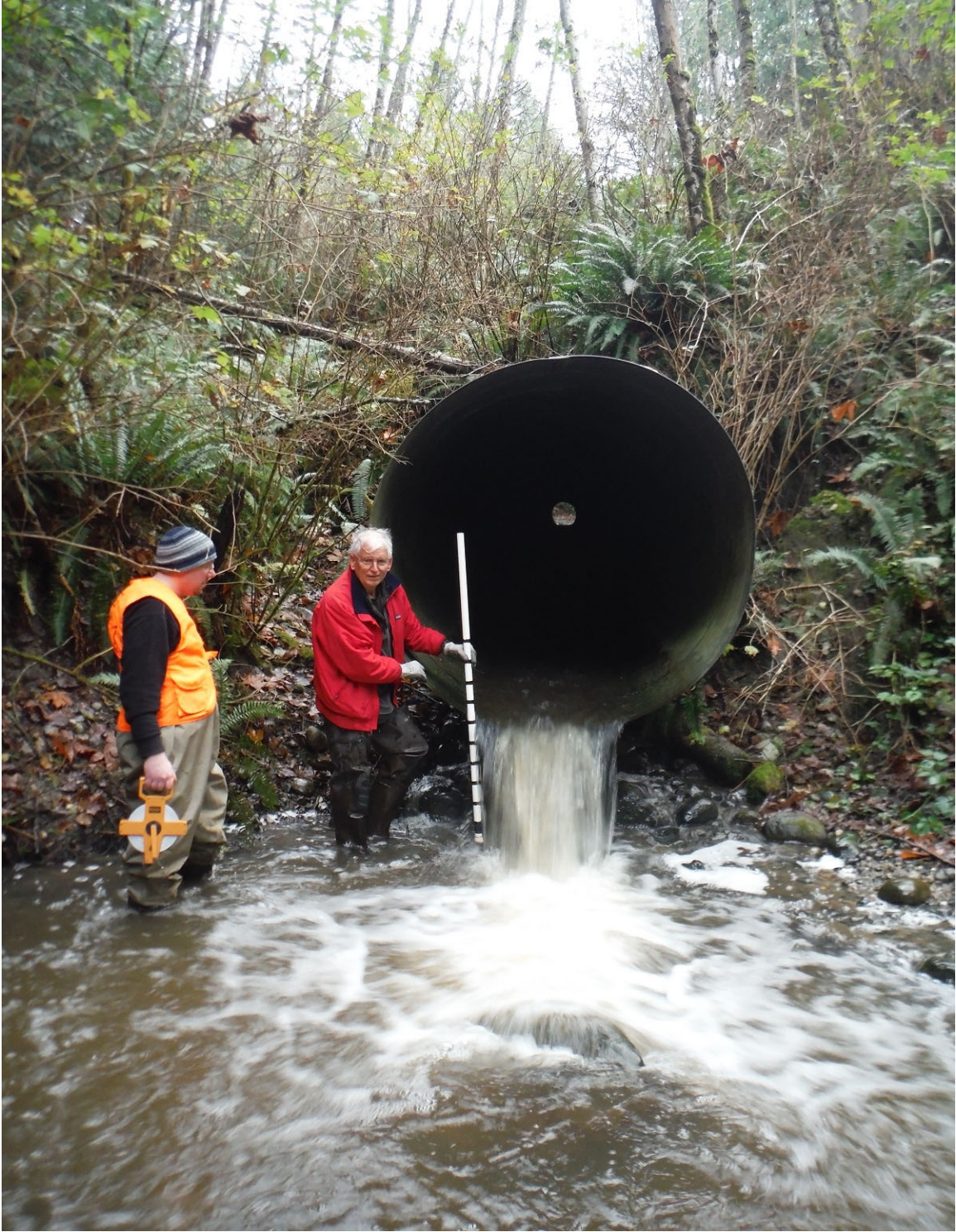
Figure 2. 2016 6 ft. diameter, 210 feet long culvert, steep, a mess, and total fish passage barrier.
